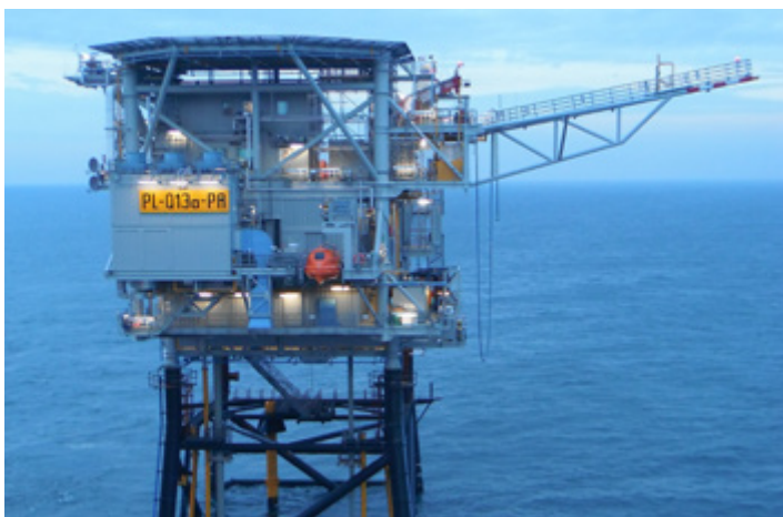
An existing oil and gas platform off the Dutch coast is being converted to the world's first offshore hydrogen platform. Electricity generated by offshore wind turbines will be used to convert seawater into demineralised water and to power a 1-MW electrolyser producing clean hydrogen.
